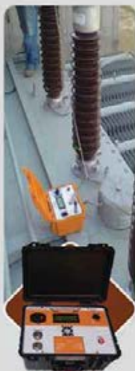
Transformer Ohm Meter
