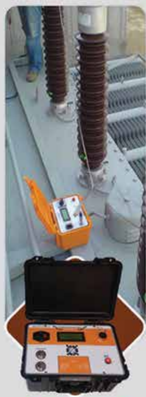
Transformer Ohm Meter
